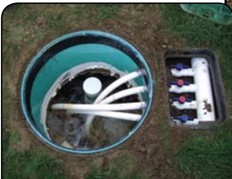
Two Cylinder Backflow Pods in operation
